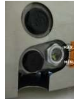
Spyhole oil tank
